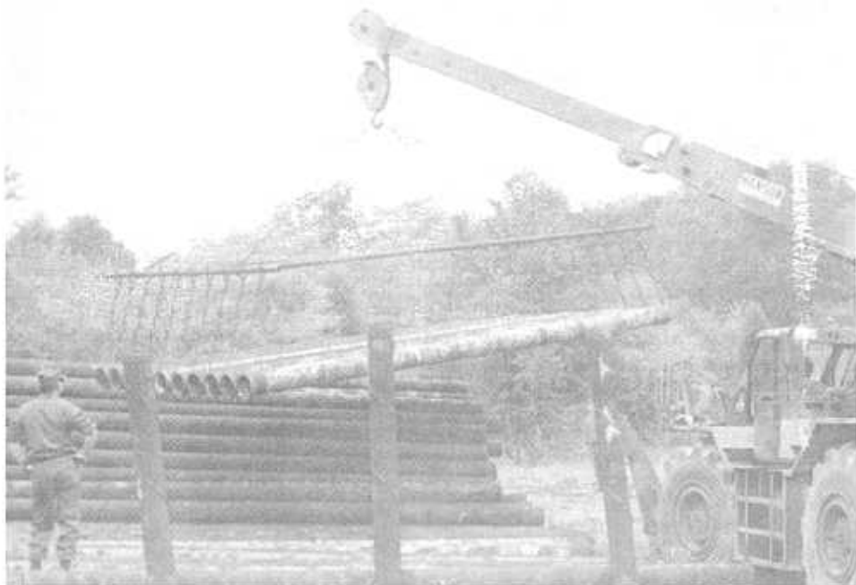
TROOPS FROM THE 201st Engineer Battalion in Ashland and Cynthiana loaded and transported pumps and pipes needed to avert a serious water shortage in three Kentucky communities.
